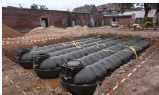
Installation NEO buffertank 3 x 20 000 l
